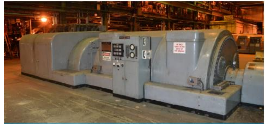
Steam turbine CHP installation at an industrial facility in New York. Photo courtesy of Recycled Energy Development
