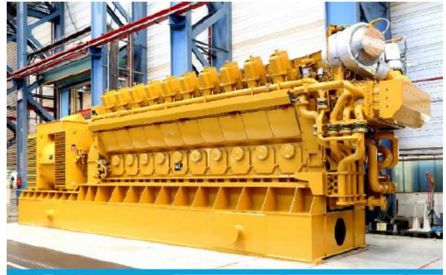
Reciprocating engine CHP installation at an industrial facility. Photo courtesy of Caterpillar.
