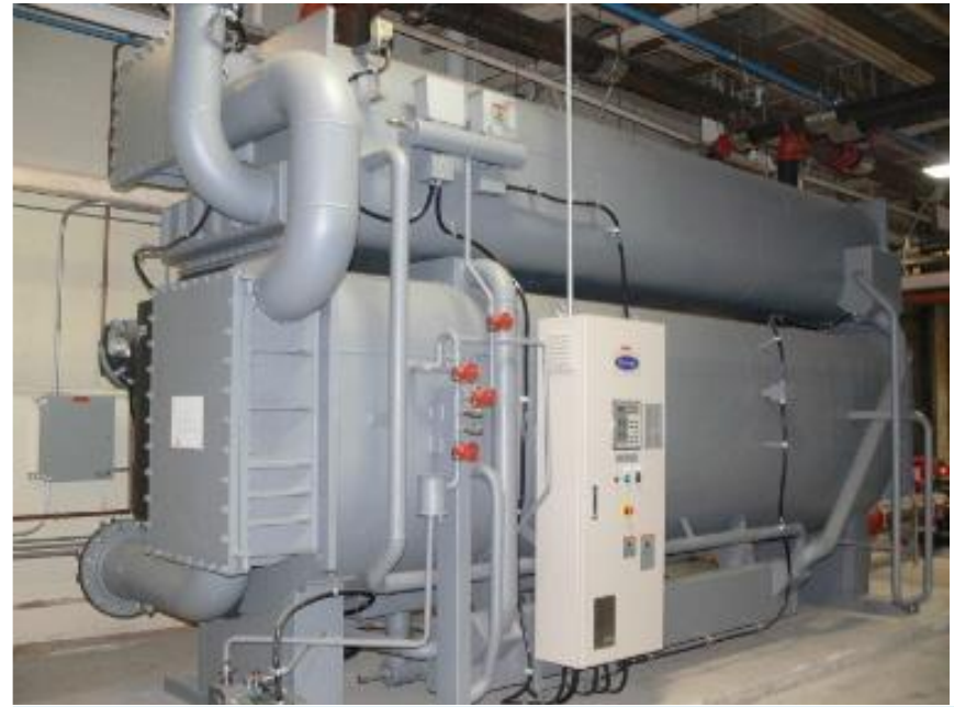
A 200-ton single-stage absorption chiller integrated with three 600 kW reciprocating engines that also provide hot water for process and space heating. The system is located at a metal fabrication facility in Fitchburg, Massachusetts. Photo courtesy of Northeast CHP Technical Assistance Partnership (CHP TAP).
