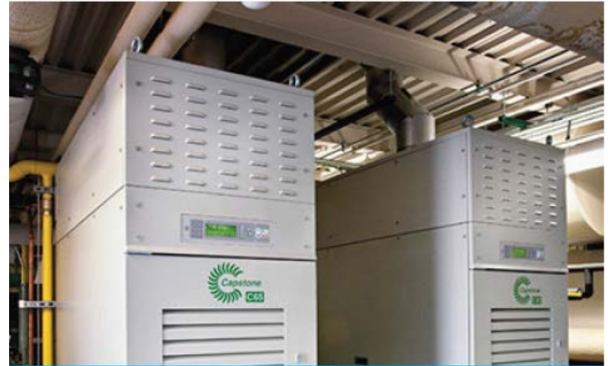
Microturbine CHP installation at a commercial facility. Photo courtesy of Capstone Turbine Corporation
