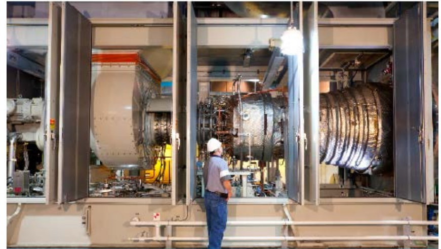
Gas turbine CHP installation at a university. Photo courtesy of Solar Turbines
