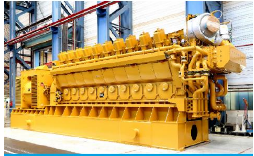
Reciprocating engine CHP installation at an industrial facility. Photo courtesy of Caterpillar.
