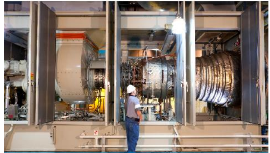
Gas turbine CHP installation at a university. Photo courtesy of Solar Turbines
